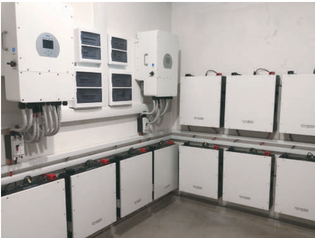
• 48kWh 10 units A48100 Lebanon
