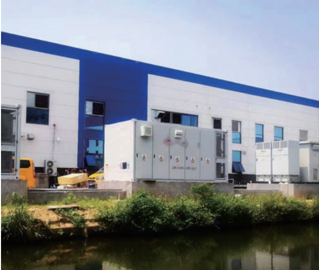
• China 5MW/18MWh DH200F Peak-shaving+PV consumption
